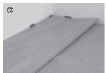
When you have interlocked the whole row on the long side and the short sides, you can lower it. Work from left to right.
